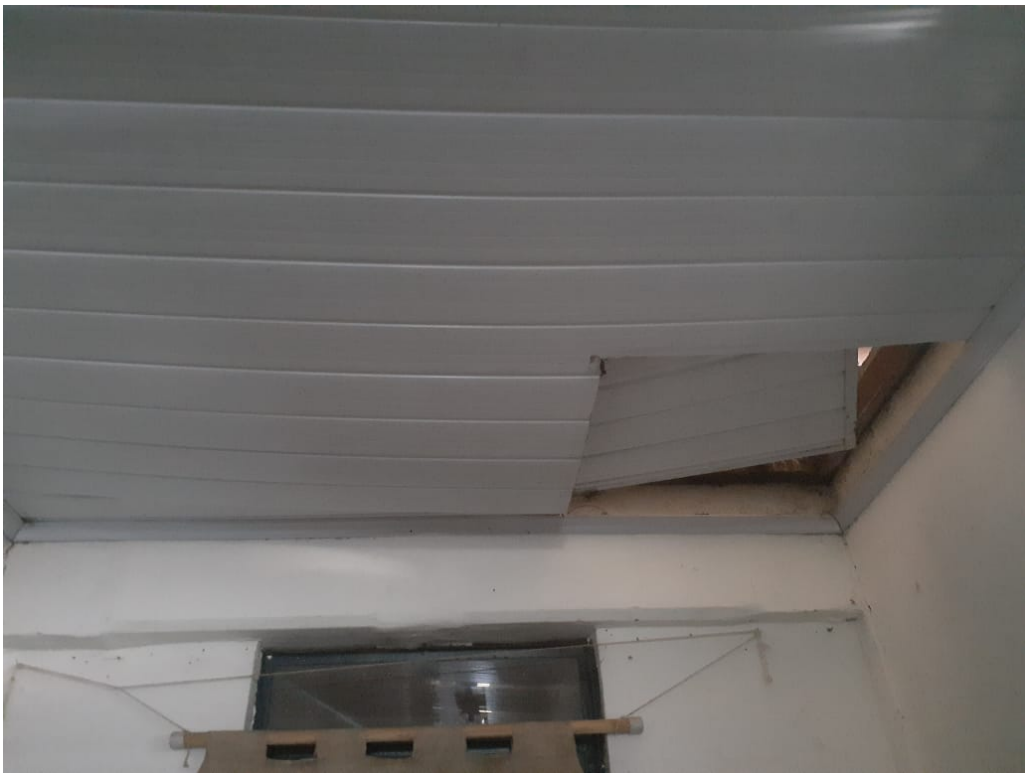
(forro de PVC cedendo)
